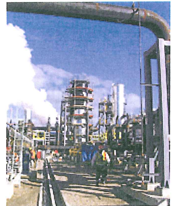
Mighty River's Kawerau geothermal plant has been successfully connected and supplied the national transmission grid.
